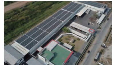
Solar panels on the roof of Thai Pigeon Co., Ltd.
