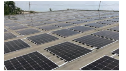
Solar panels on the roof of PT Pigeon Indonesia
